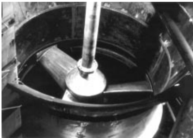
Fig. 7 C110 3.2 meter impeller in 50 ft tank
